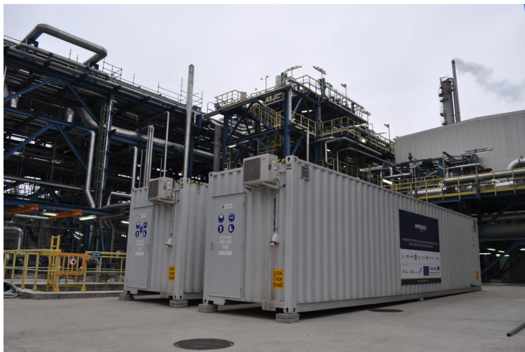
The Improved containers at the ureum plant at Yara Sluiskil
